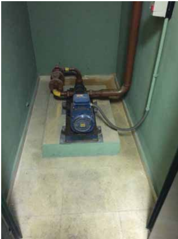
SALA BOMBAS GASOIL
